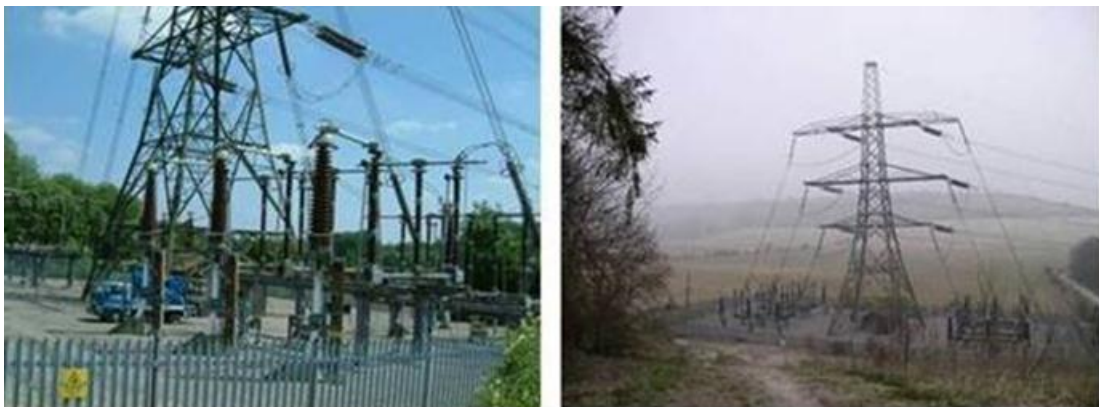
Figure C.5: Cable Sealing End Compounds
